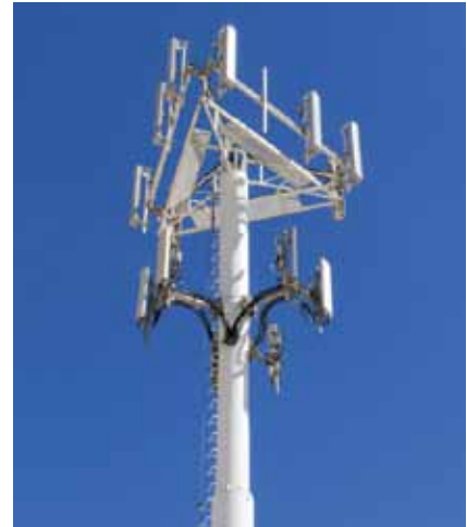
Typical cell tower with antennas configured to provide service to equally divided sectors.
